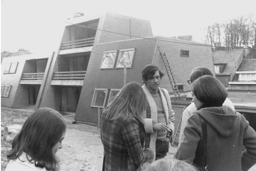
Photo of the building site of the Abreuvoir project, 1973, Bruxelles © Archive Françoise Wolff.
