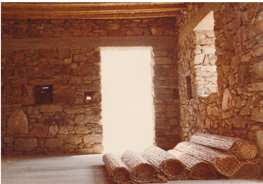
Villa T, under construction. Rolls of raffia used for the ceiling insulation, 1982. Courtesy Katerina Tsigarida Archive.
